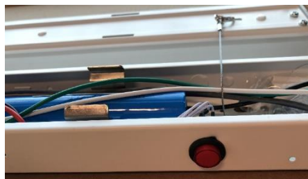
Emergency Test Button
